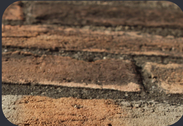
Figure 2. Damage over brick and mortar
