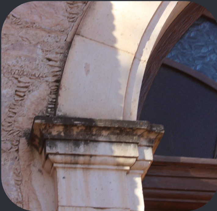
Figure 1. Damaged quarry stone
