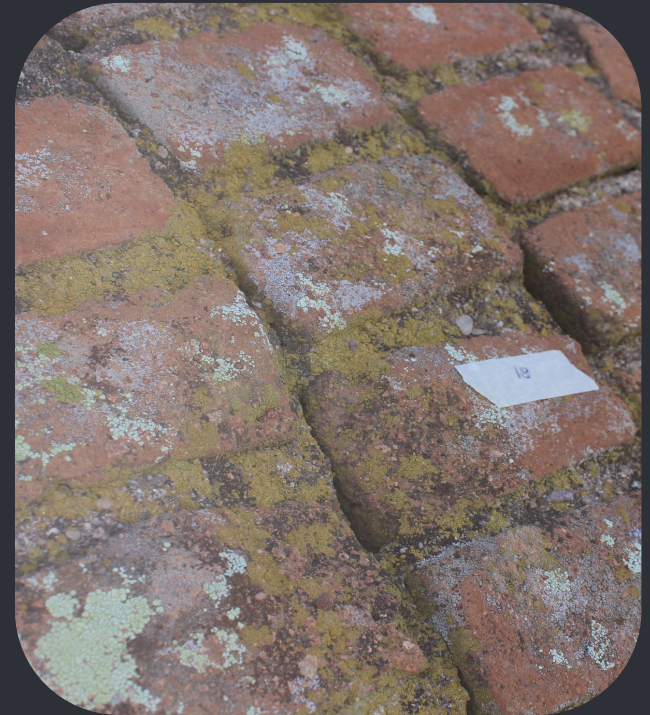
Figure 4. Damage over brick (mustard lichen)
