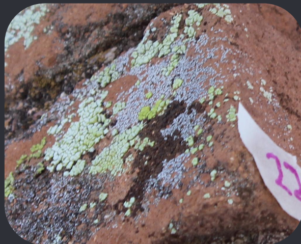
Figure 6. Damage over brick (gray lichen)
