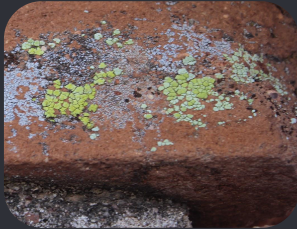
Figure 5. Damage over brick (green lichen)
