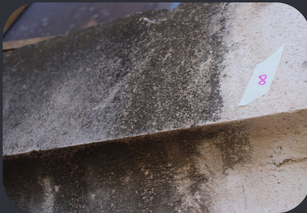
Figure 3. Damage over quarry stone
